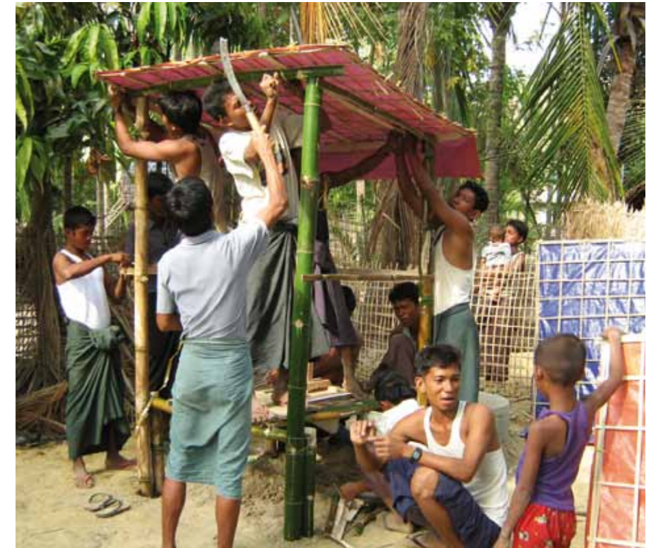
With guidance from the Malteser International staff, the village residents build latrines for their families as well as for schools and other public facilities.
