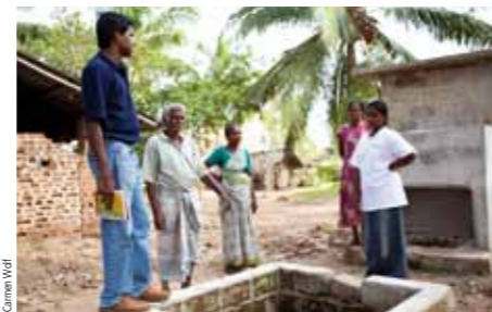
New household latrines and sanitary facilities for schools and health centres are being installed in 46 villages.
