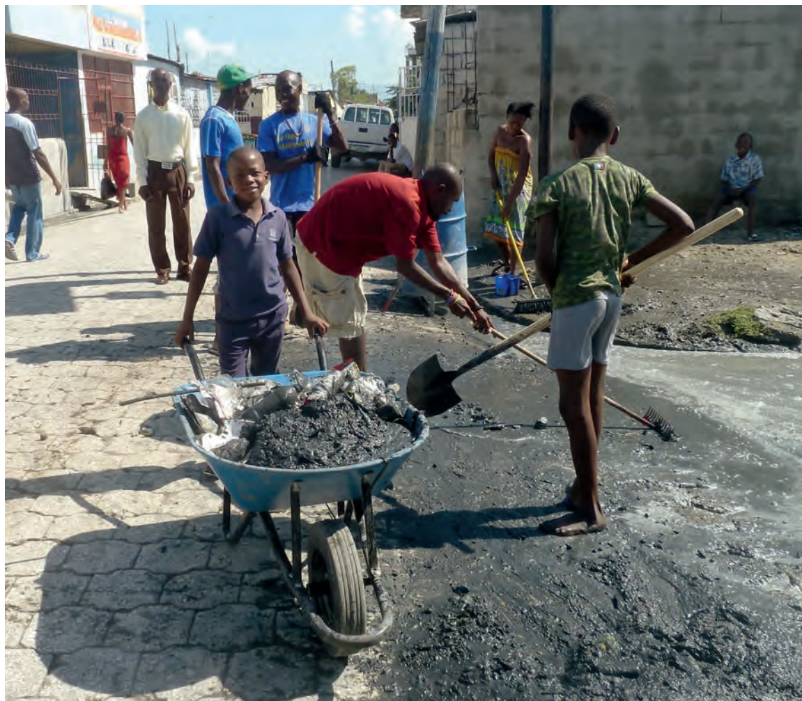
Working together to tackle the mess: in Cité Soleil volunteers work to clear garbage from waste-water channels.
